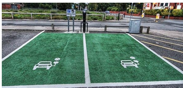
Figure 38: Example of electric car charging power point
